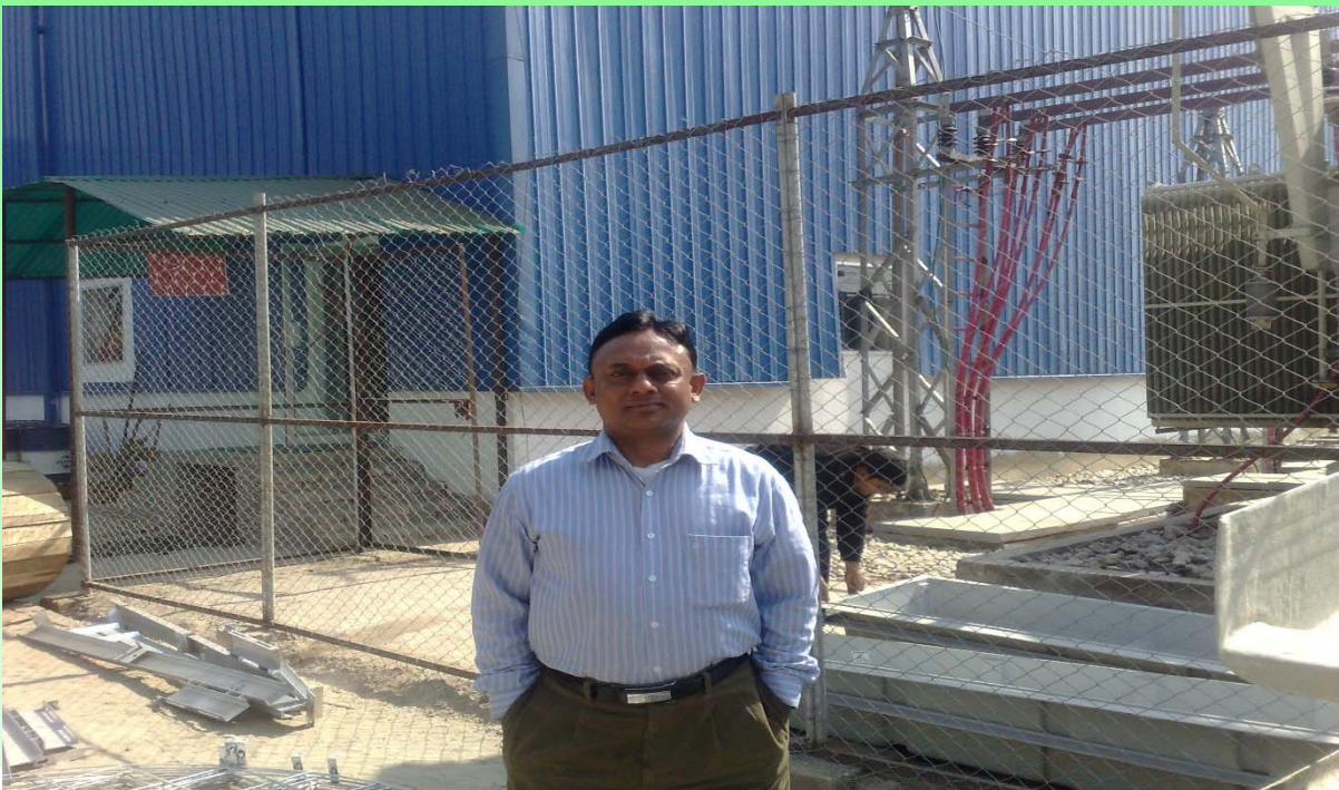
Site Supervision by Engr. Rafiq Ul alam Power Plant at Bogra Unit MWM
