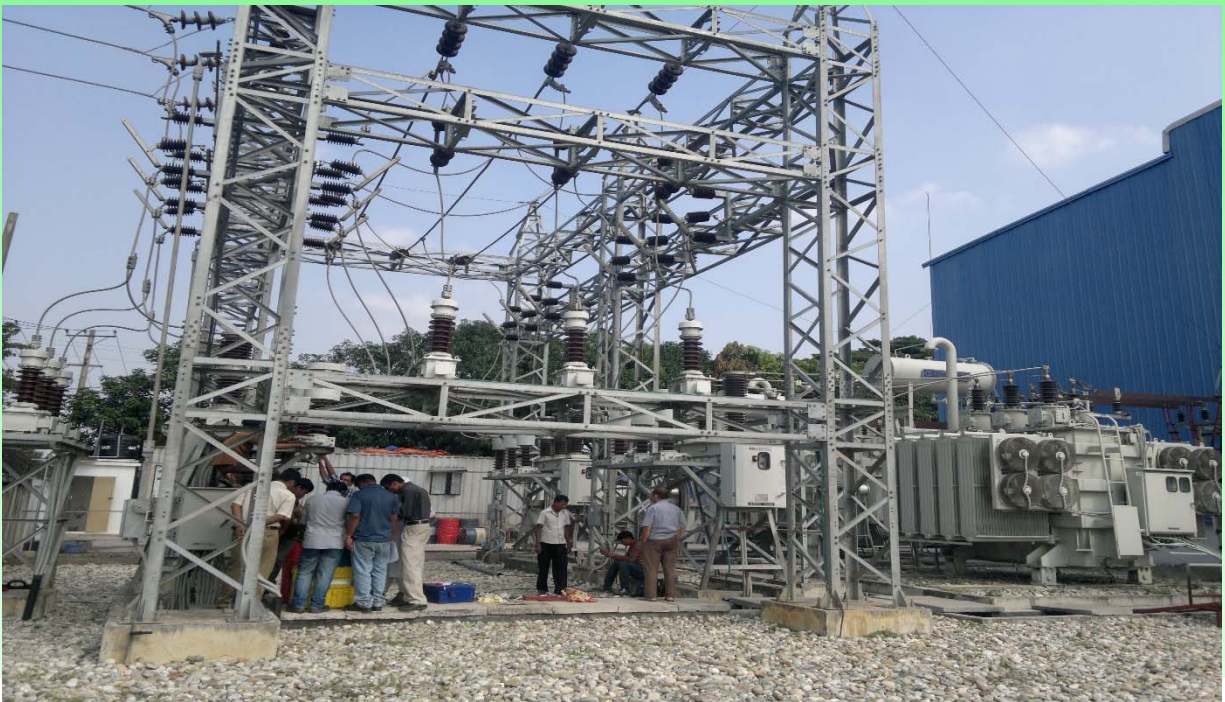
GRID SWITCH yard of 20 MW Energy Prima of HOSAF GROUP
