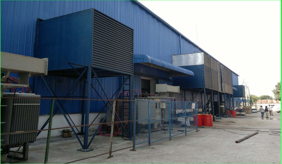
20 MW Rental Power Plant at Bogra Unit MWM
